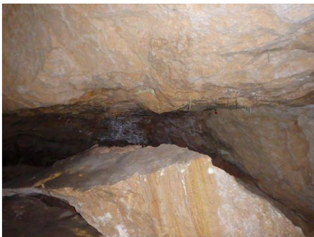
Figure 59: The northernmost part of the condensation sheet at location 2. Photo Rob Foulds
